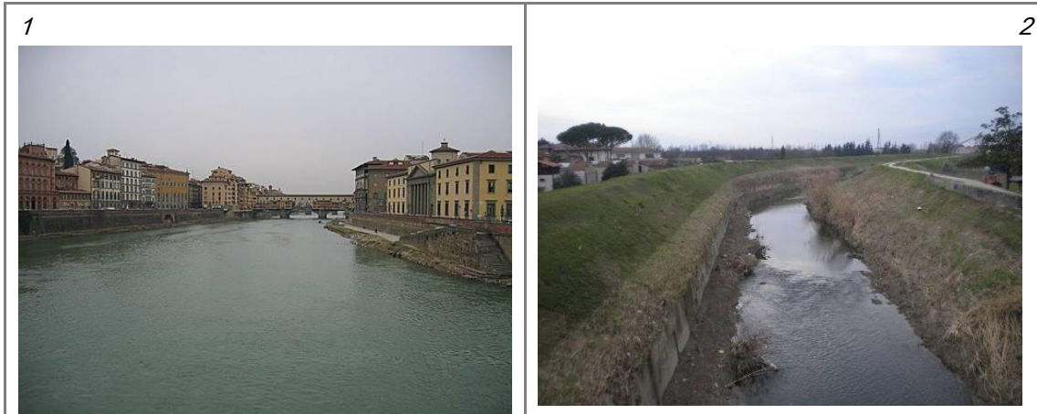
Figure 63 Cases of bank-edge levées occurring for most of the reach, for which an additional score of 6 or 12 (depending on the % of the reach length) is added.
