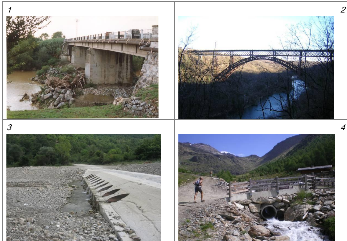
Figure 56 Crossing structures. (1) Bridge with interference on fluvial dynamics; (2) crossing structure unrelated to the fluvial corridor; (3) ford with culverts; (4) culvert.
