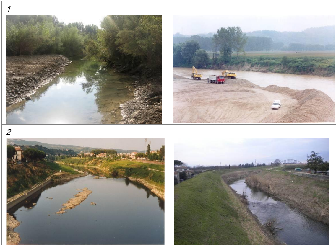
Figure 32 Alteration of cross-section variability in partly- and unconfined channels. (1) Cases of partial homogenization of the cross-section due to interventions. (2) Cross-section homogeneity extended for long reaches due to excessive artificiality.
