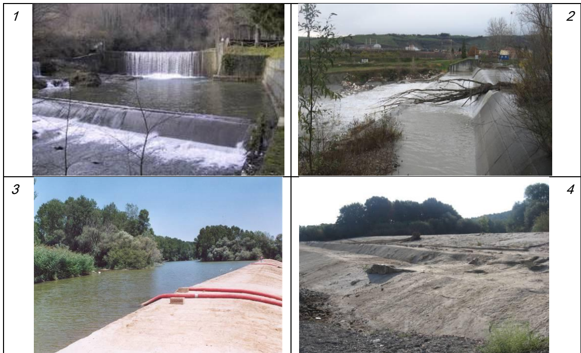
Figure 49 Transversal structures of alteration of sediment discharges in hilly and lowland areas. (1) Consolidation check dam; (2) abstraction weir; (3) not filled abstraction weir; (4) filled abstraction weir.
